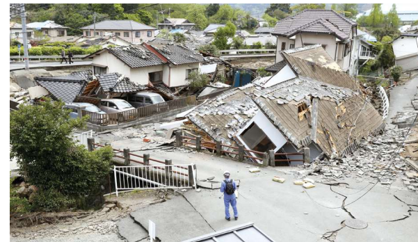
Many houses collapsed due to strong shaking in the Terasako district of Mashiki Town, Kumamoto Prefecture [Photo provided by Kyodo News]
