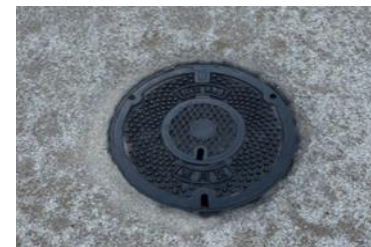
④防火水槽
